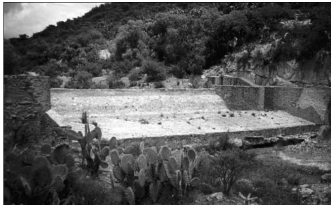
Figure 1. Hydraulic infrastructure from the hacienda times still in use.
